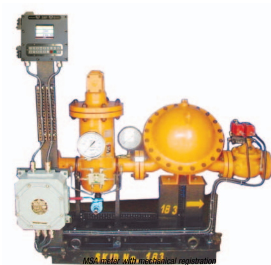
MSA meter with mechanical registration
